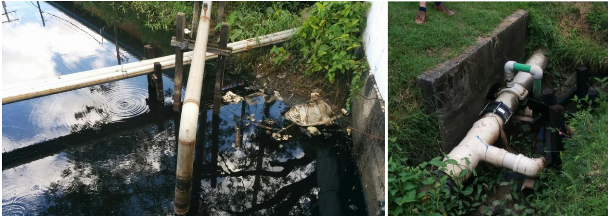
Figure 56 Drainage system blocked by other works (Joost Remmers, August 2016)
