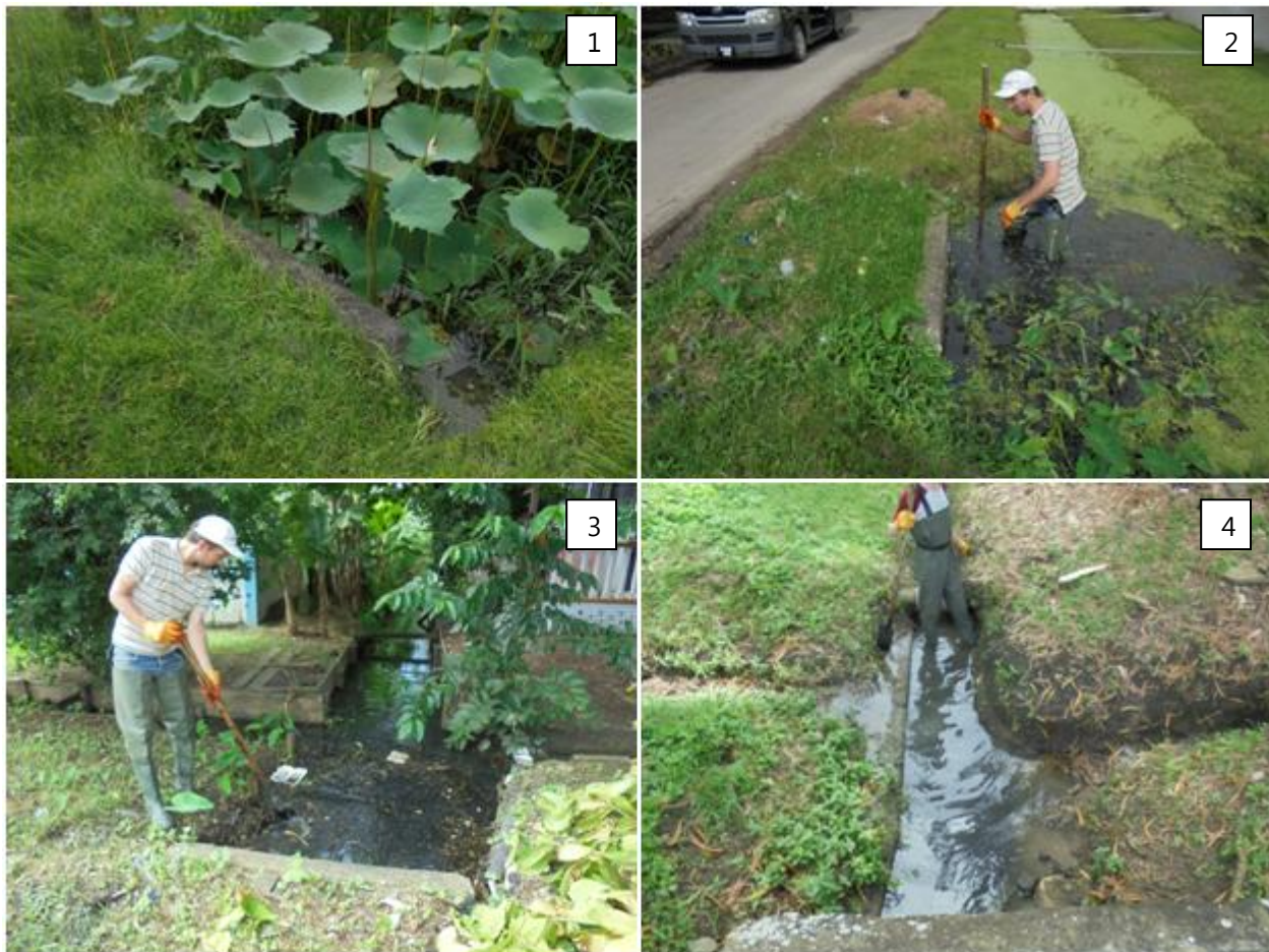
Figure 12 State of channels in front of culverts
