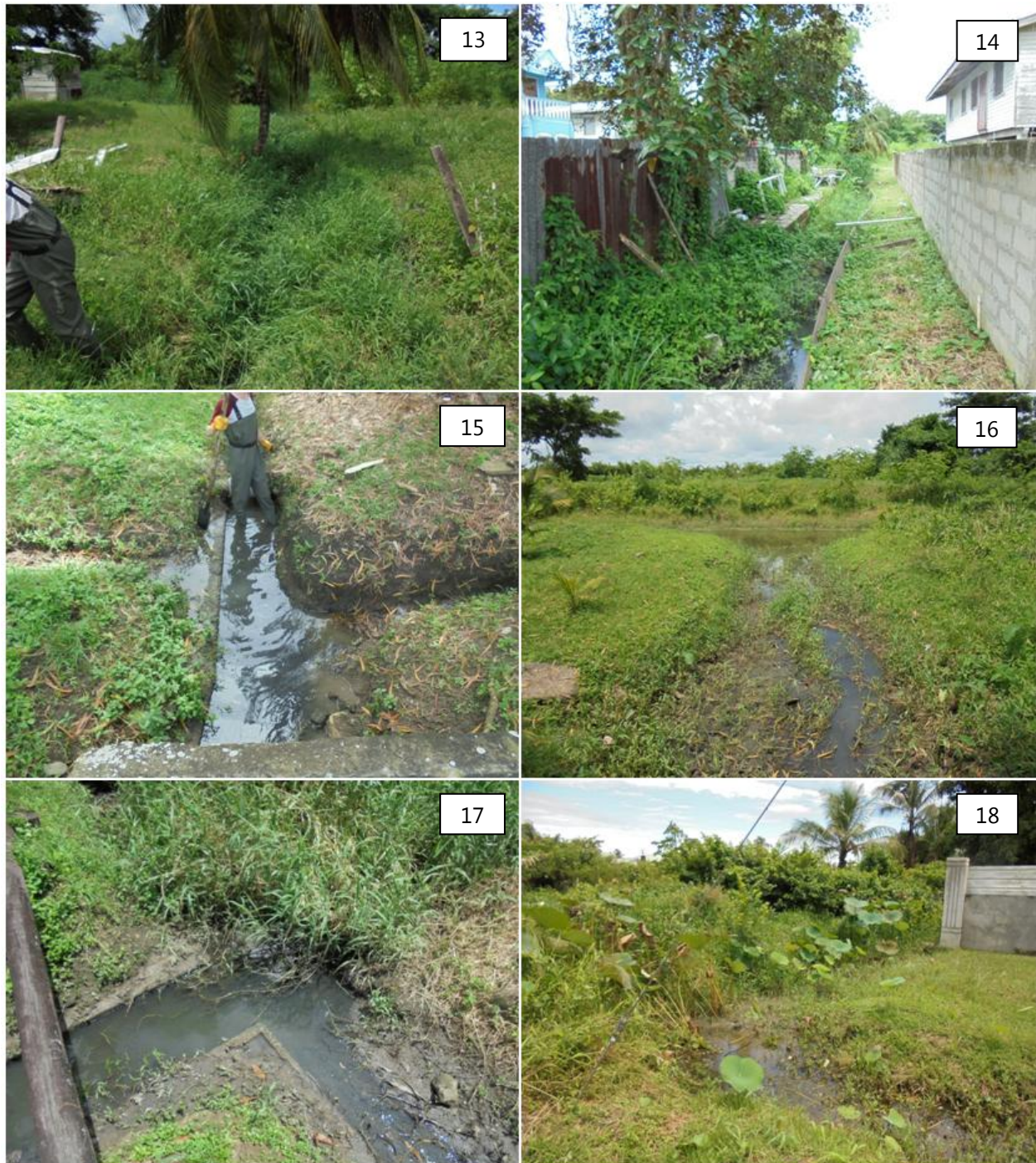
Figure 77 Illustrations on local drainage system (3) (Ruben van Montfort, August 2016)
