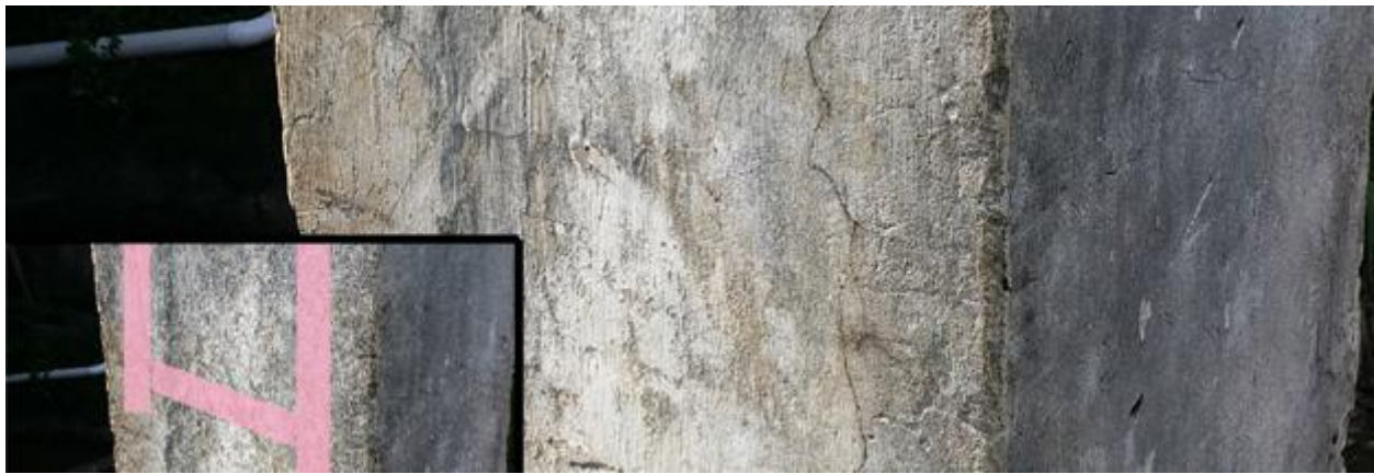
Figure 52 Example of a rebar crack worth an 8 on the inspection form (Peter Vijn, August 2016)
