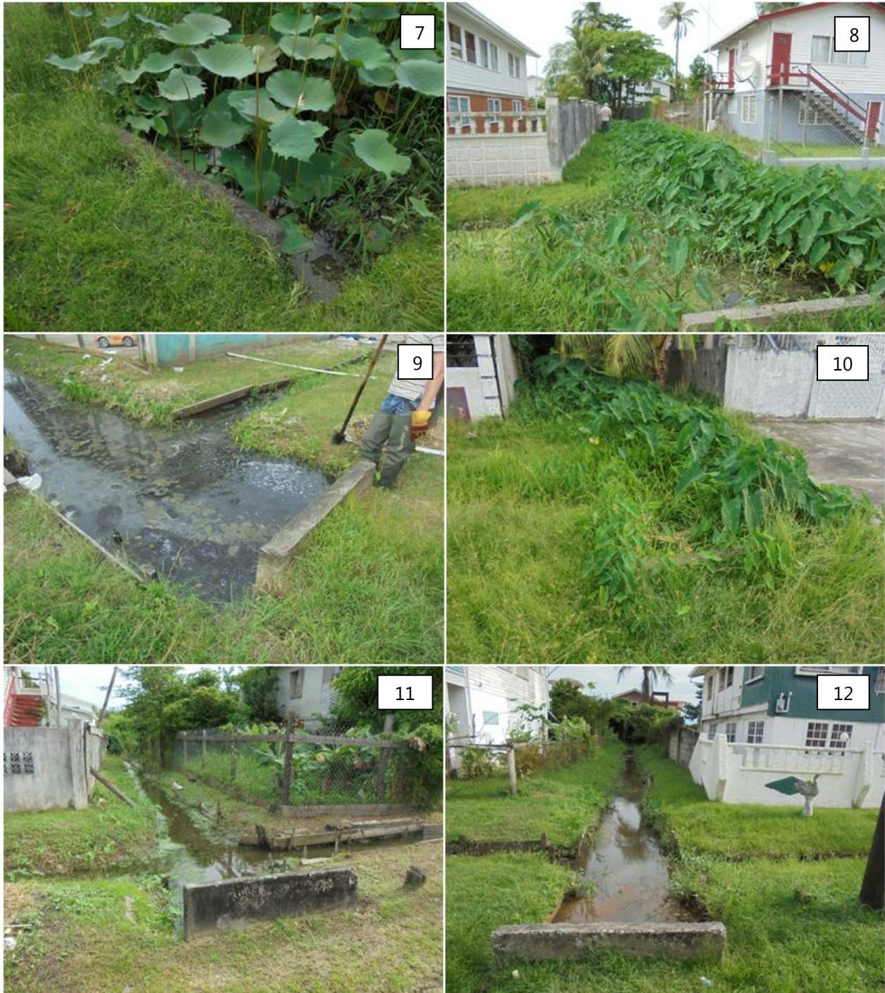
Figure 76 Illustrations on local drainage system (2) (Ruben van Montfort, August 2016)
