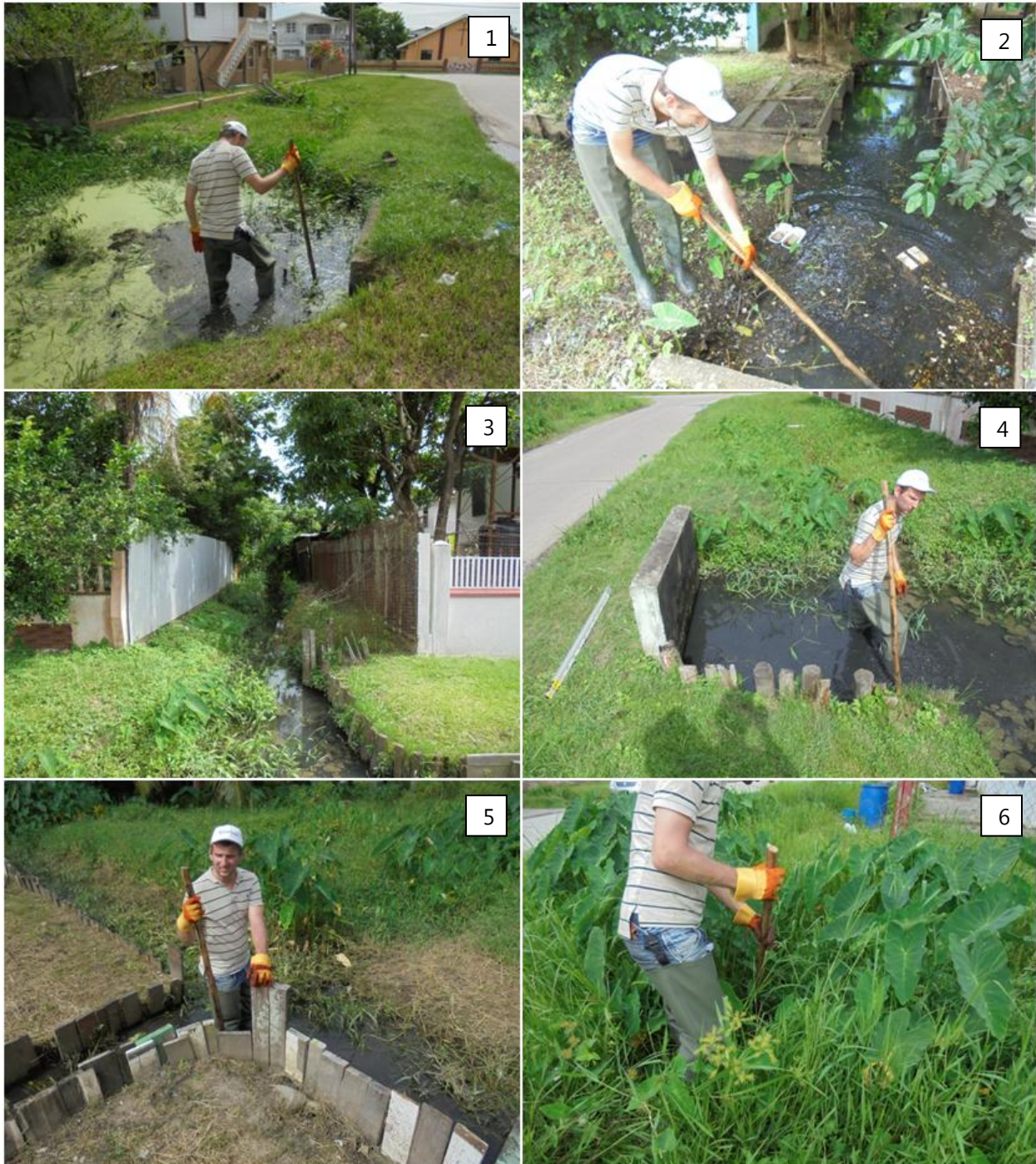
Figure 75 Illustrations on local drainage system (1) (Ruben van Montfort, August 2016)
